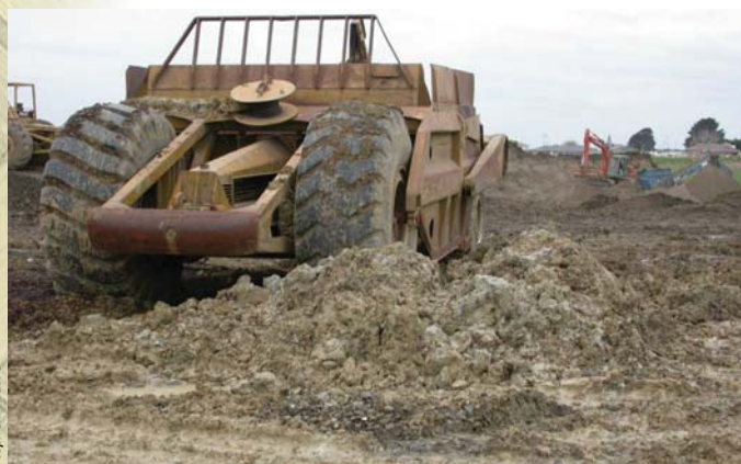
■ The opposite of LIUDD: a large new subdivision development in Auckland. Major earthworks such as these cause extensive soil damage.
