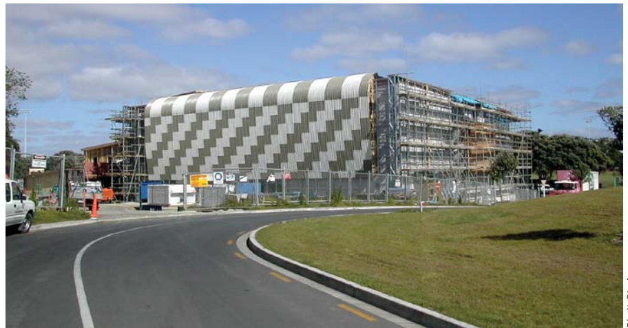
■ Principles in practice: Landcare Research's new "green" building, currently under construction on Auckland University's Tamaki campus. This energy-efficient building was constructed according to LIUDD principles and has rainwater tanks to help conserve water.
