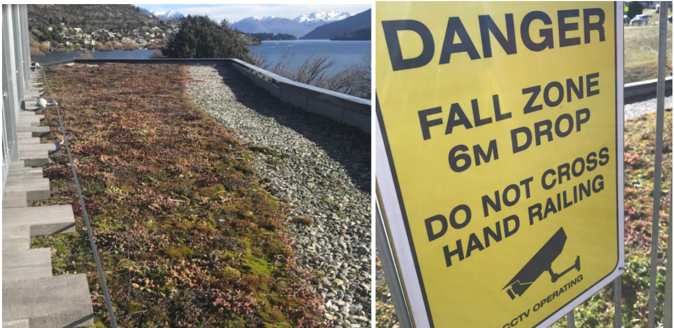
Remarkables School decking with safety cable, sedum carpet and adjacent pebbled drainage strip which also minimises maintenance near the edge. Warning signs, locked gate and camera surveillance are used to discourage roof access.
