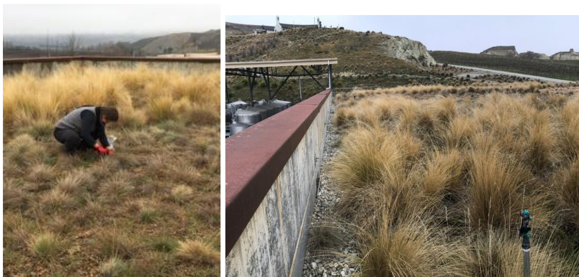
Mt Difficulty roof at age 6.5 in early spring before sedums flower; the right photo shows the gravel drainage edge that runs along the concrete parapet with the restoration area that includes the hill slopes up to the restaurant (2018)
