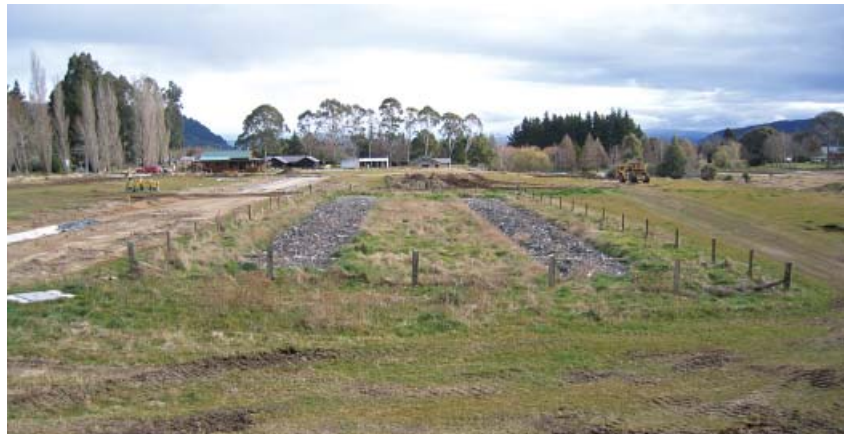
Denitrification beds at Kinloch filled with sawdust and bark. These beds remove nearly all the nitrogen from wastewater passing through them
