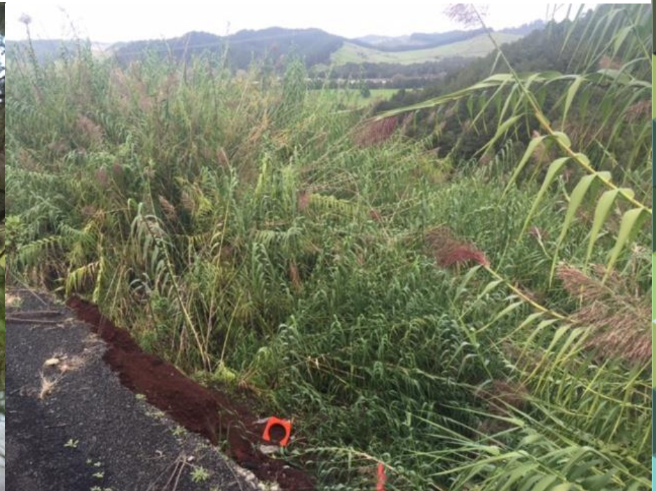
Giant reed planted to stabilise a road edge at Moerewa has spread across the whole hillside
