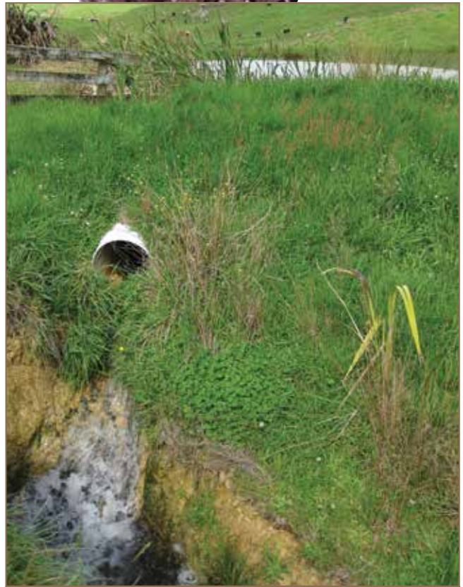
Perched culvert preventing fish passage. Raglan, Waikato. Photo: Monica Peters, NZ Landcare Trust
