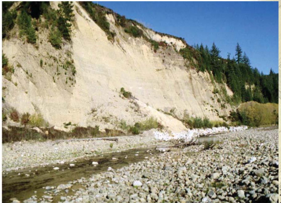
■ Bank erosion in the Motupiko River, which carries sediment into the upper Motueka River.
