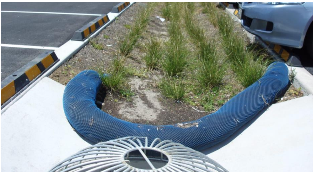
Park n Ride swales (2012 photo – should not plant in straight lines like this)
